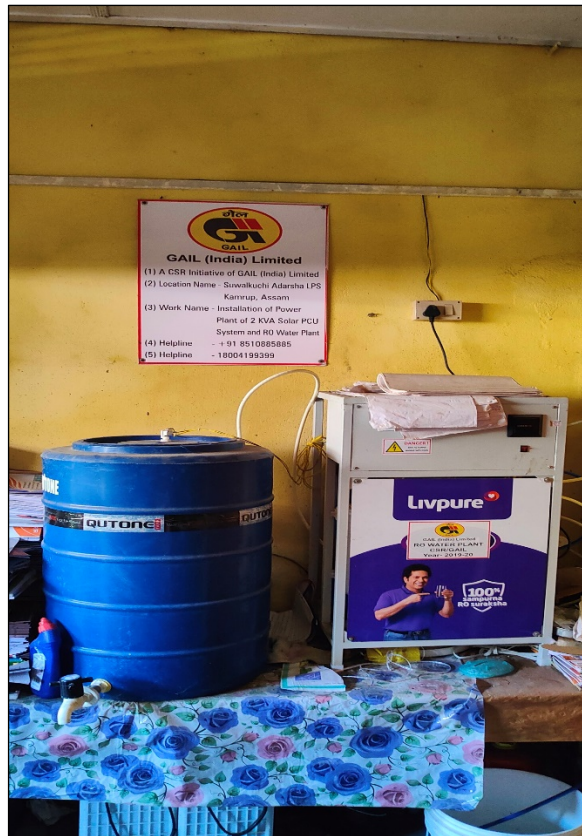
Figure 6: GAIL Branding for RO water purifier plants in schools
