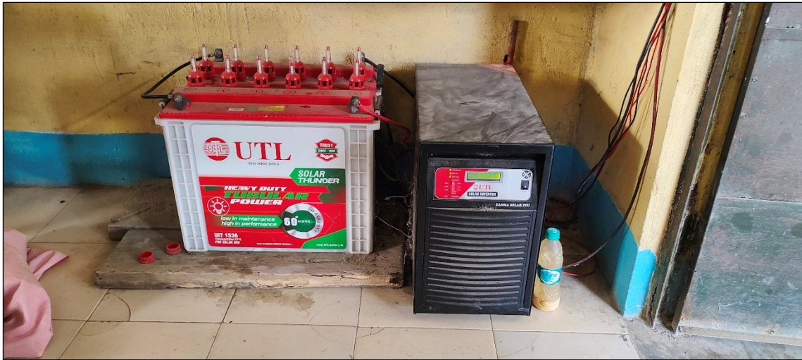
Figure 16: Solar hybrid power pack installed in one of the schools
