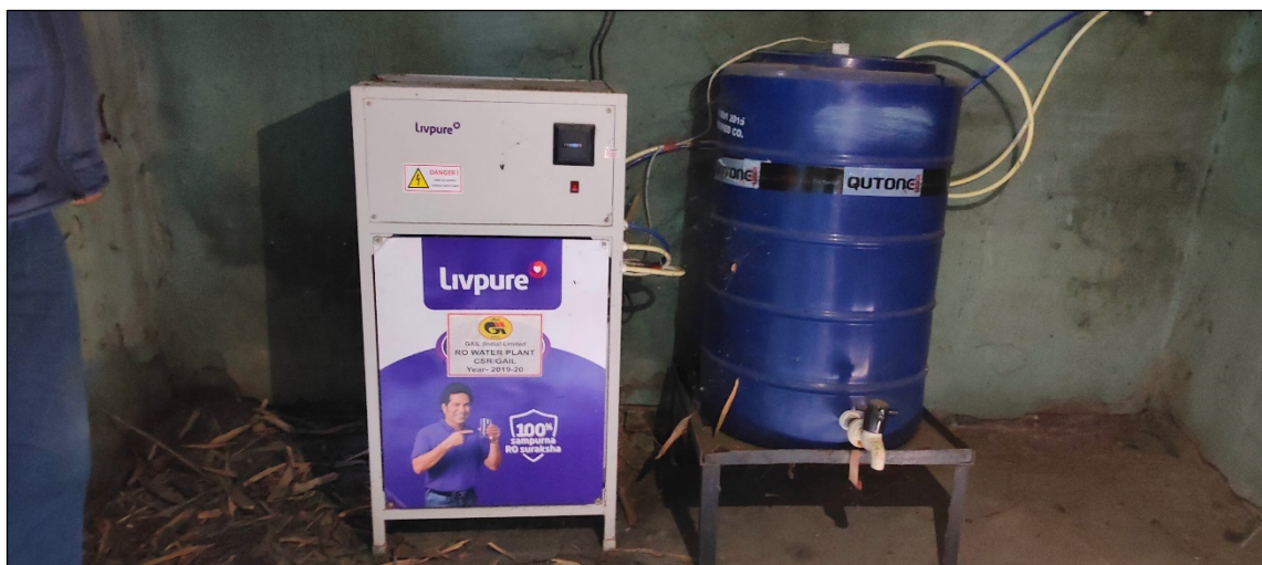
Figure 10: RO water plant in one of the schools
