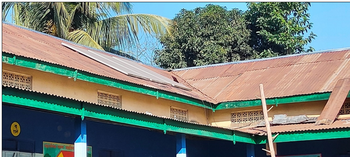
Figure 14: Solar panels installed on the rooftop of one of the schools
