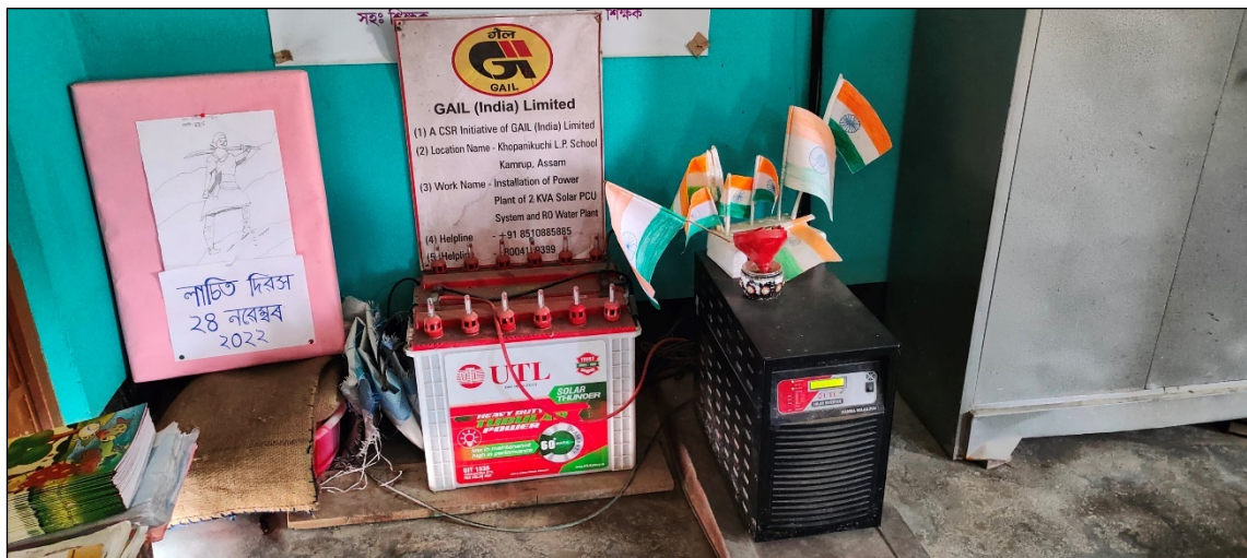
Figure 17: Solar hybrid power pack installed in one of the schools
