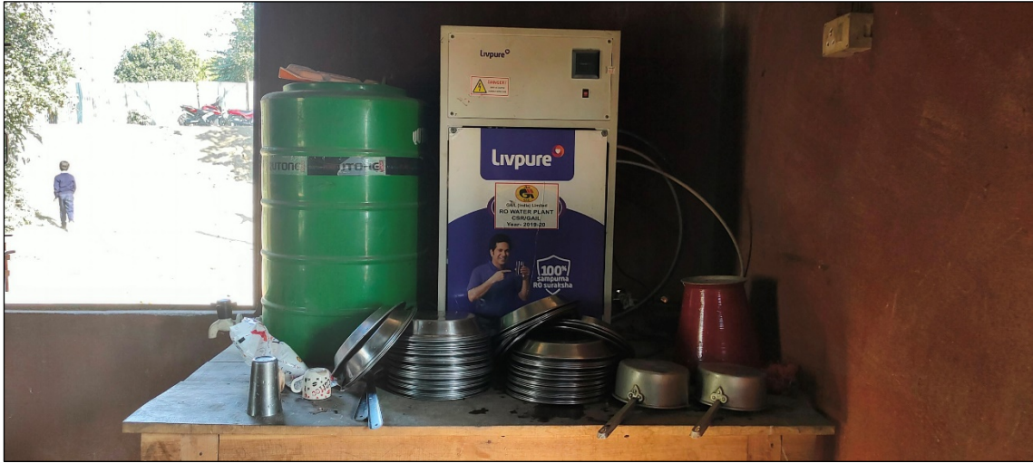
Figure 7: RO water plant in one of the schools
